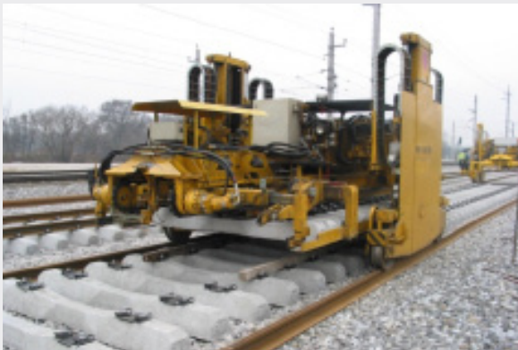
Temporary storage of the sleepers on track then transport and lay Sleeper in track with second unit
