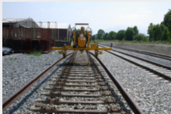
Continuous, steady placement of rails on the sleepers at the requirement gauge with ROTHREAD
